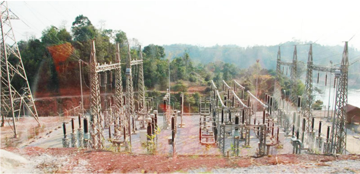
Theun-Hinboun Switchyard 2 image below:
